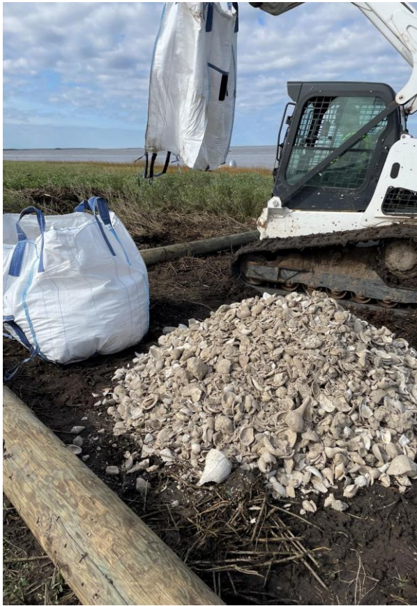
Various images of moving shell, preparing site, timber frame construction, shell backfilling and geocell fabric use.
